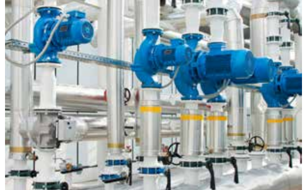
Pressurization Motors and Pumping Systems
