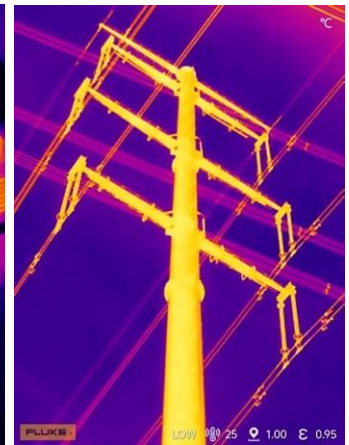
Power transmission lines
